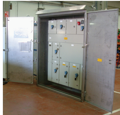
Functional Supply Point (FSP) Kiosk
